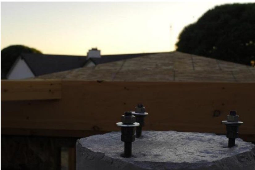
Concrete Pier Leveling bolts.jpg
